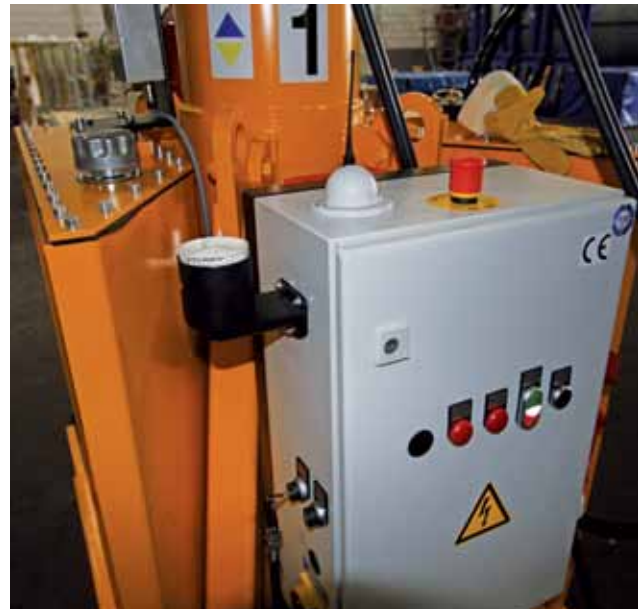
Figure 7: Electric control cabinet for a leg of the lifting facility
