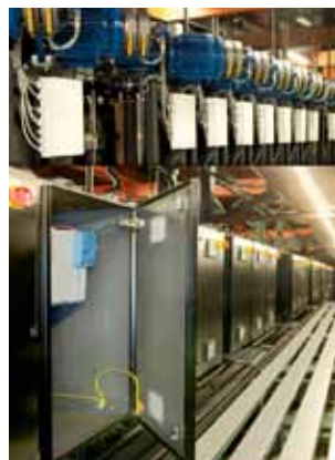
Figure 3: The safe control solution includes customized enclosures for each of the more than one hundred drives in the upper and lower machinery
