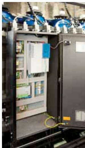
Figure 1: Each enclosure contains one ICU computer by Unican (bottom left) and an SK 535 frequency inverter by Nord (top right)
